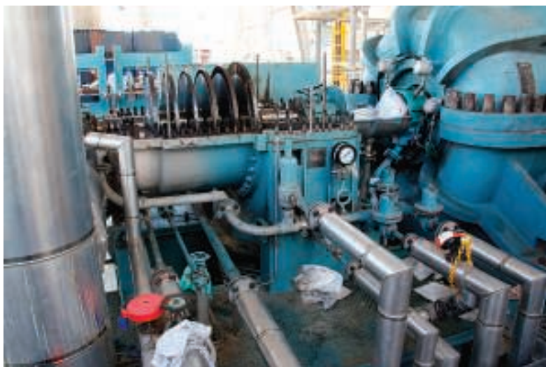
FIGURE 1. Shown here is a steam turbine dismantled for repair. This is the driver of the centrifugal compressor
