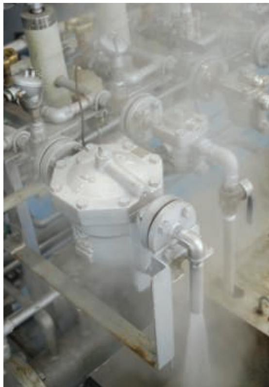
FIGURE 1. Effective steam traps keep heat in the system to optimize production rates and heat quality, and they also discharge condensate to provide for system safety and reliability. Major problems can occur if condensate is not readily drained from the system
