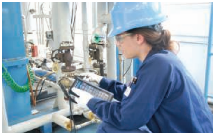
FIGURE 3. Accurate and regularly sustained diagnosis of steam traps’ operating conditions is essential to determining the population’s current health (state of the population). Once failures are identified, the information is valuable for allocating resources to restore all condensate discharge locations to an “as designed” operating condition for safety and reliable performance
